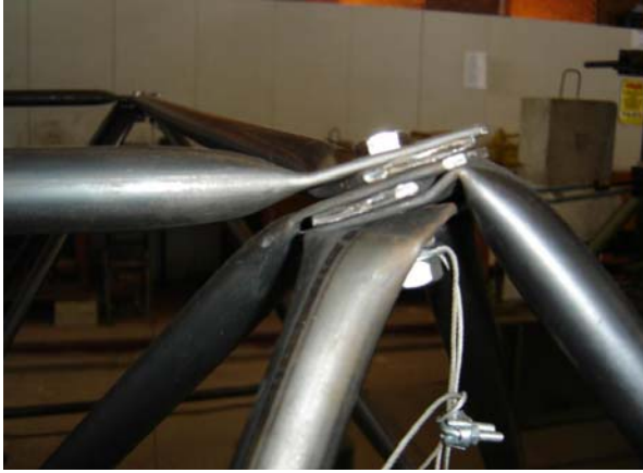
Figura 9.2 – Colapso local ( P=25\text{kN} )
