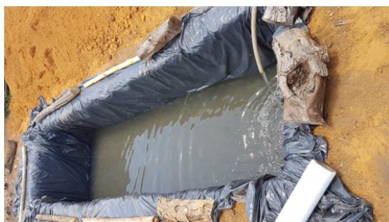
(a) Trench filling up with water.
