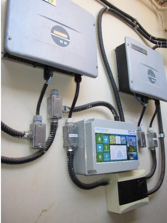
Figure 24. View of metering and monitoring equipment installed by Solar Energy do Brasil in CEACA-Vila, Source: C.A.G.Garcez Date: February 2015
