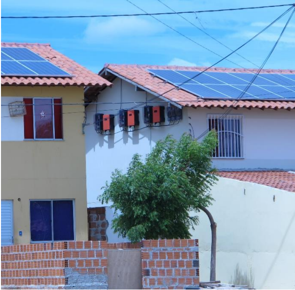
Figure 19. View of solar PV panels and inverters installed in Juazeiro Source: C.A.G.Garcez Date: November 2013
