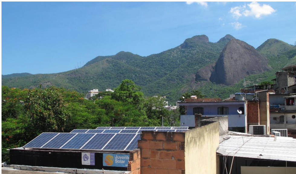
Figure 23. View of rooftop solar-PV installation in Morro dos Macacos, Source: C.A.G.Garcez Date: February 2015
