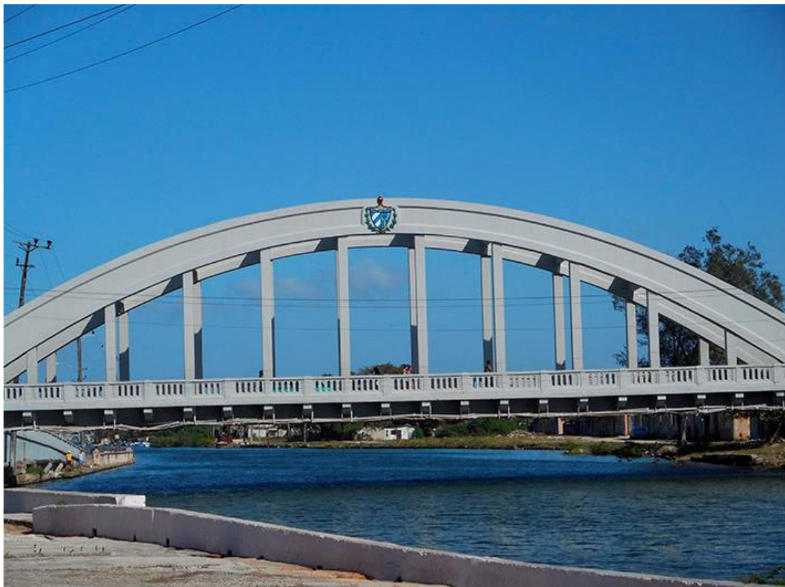
Picture 21 - Tirre Bridge above the San Juan River that separates Pueblo Nuevo from downtown Matanzas and La Marina, Matanzas, Cuba.
