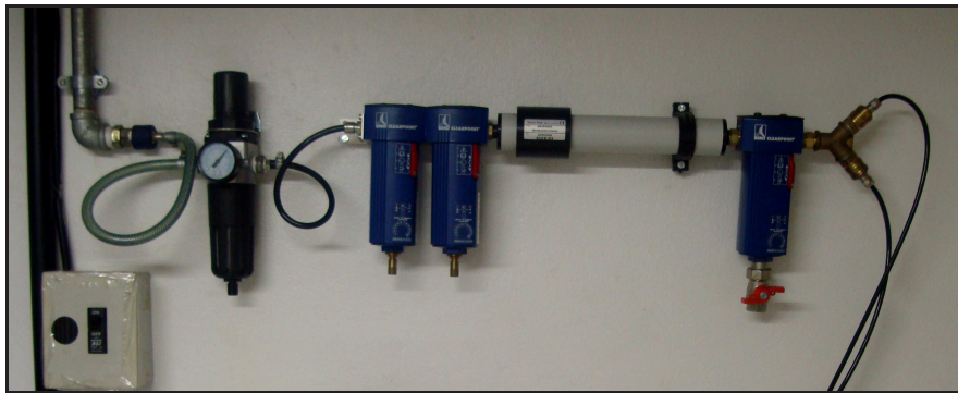
Figure 7.9: Filters used to clean and dehumidified the compressed air from the Schulz compressor
