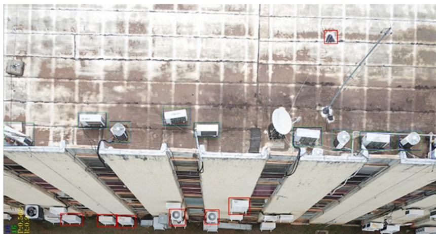
Fig. 15. Detection errors of condensers on the facade by the Fovea network.
