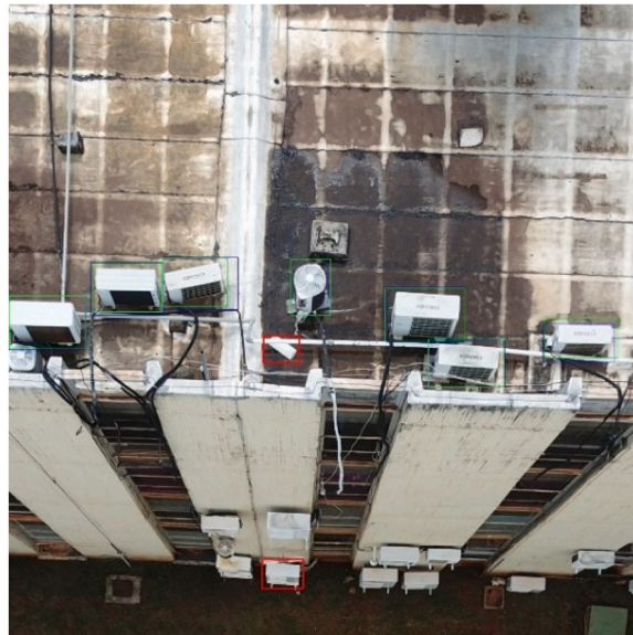
Fig. 16. Pooling of water in the region of the condensers.
