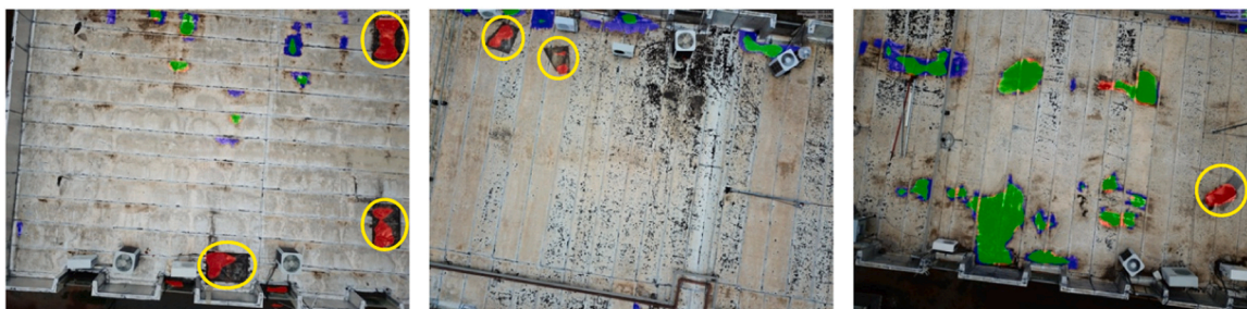
Fig. 19. False positive segmentation of rubbish on the flat roof - FCN with Adagrad optimizer and a learning rate 1e-4 .
