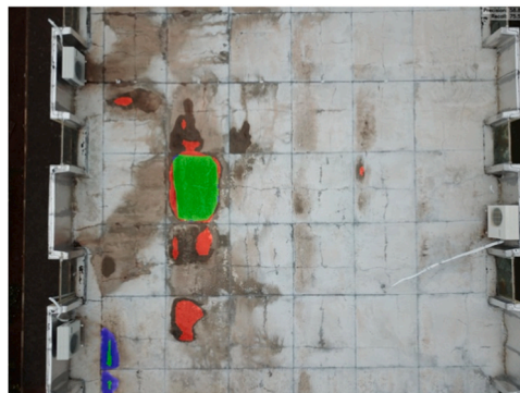
Fig. 16. Light and dark moisture stains on mechanical protection with mortar - FCN optimized with Adagrad and rate of 1e-4 .
