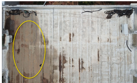
Fig. 3. Light moisture stains on the flat roof after rain.
