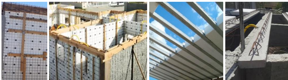
Figure 2. 3 - Execution of slab directly supported on sandwich wall panes cast in situ.
