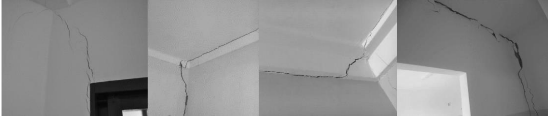
Figure 2. 4 - Cracks found in the connection of wall-slab of houses without distribution beam at wall top.
