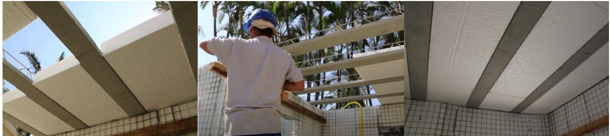
Figure 2. 2 - Execution of slab directly supported on sandwich wall panes cast in situ.
