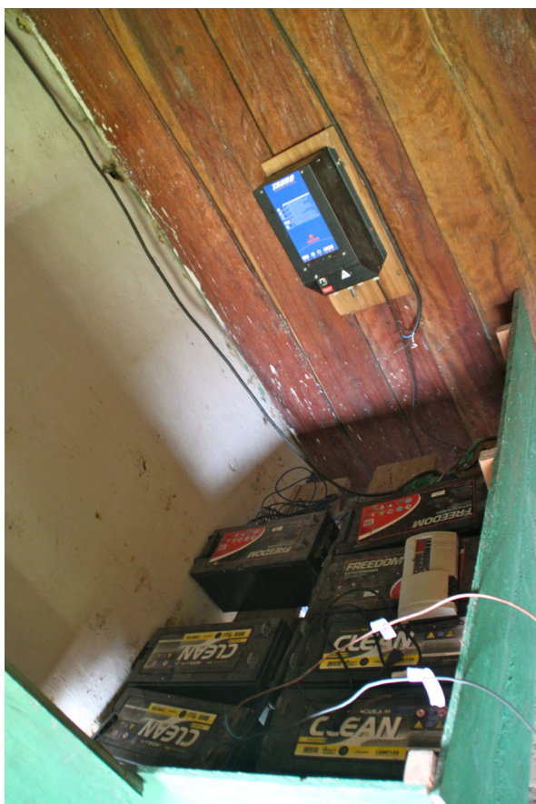
Batteries used to store solar energy at Pamáali School
