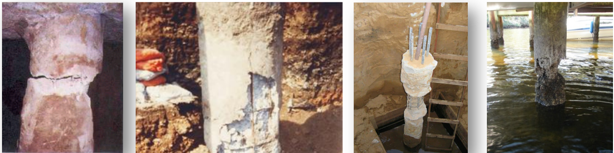
Figure 2.5. Some actual examples of damaged piles. (Freitas Neto, 2013).
